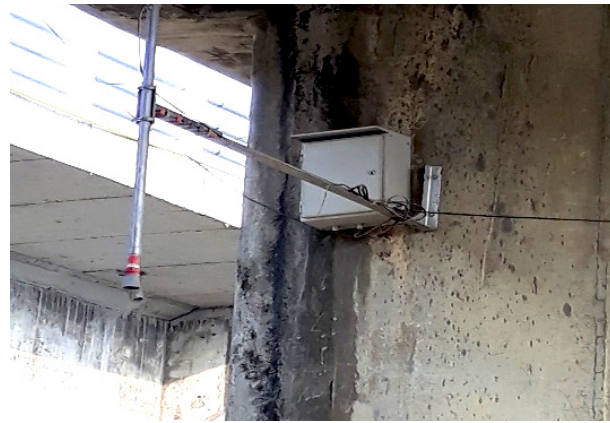
AN EARLY WARNING SENSOR IN RATU BRIDGE, BARDIBAS, NEPAL.
