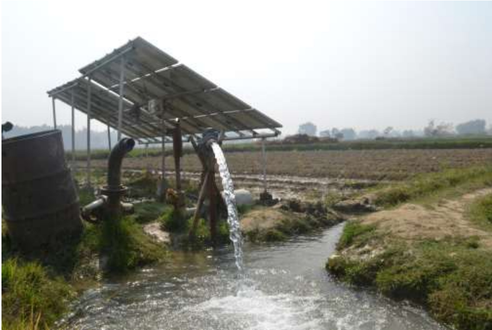
2HP system in Hardiya
