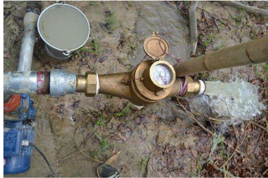
Flow meter installed to measure discharge
